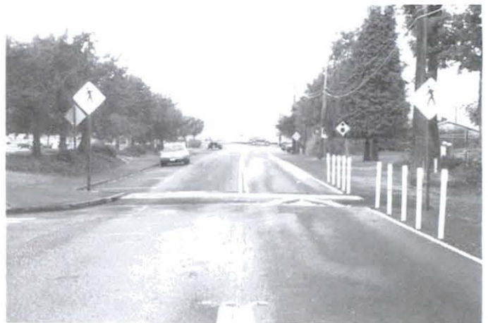
A project completed in March 2000 was a raised crosswalk with signage improvements at the intersection of Redondo Way South and 4th Place South.
